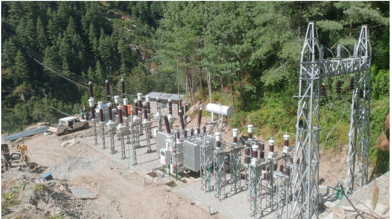
Figure 8: Completed Interconnecting switchyard at 300 m U/S from Beni Powerhouse.
