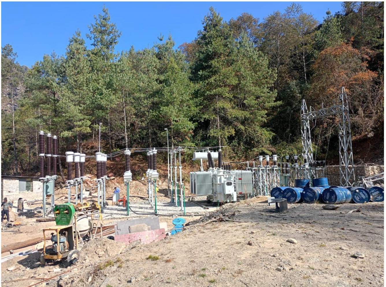
Figure 9: Interconnecting switchyard ready for Charging.
