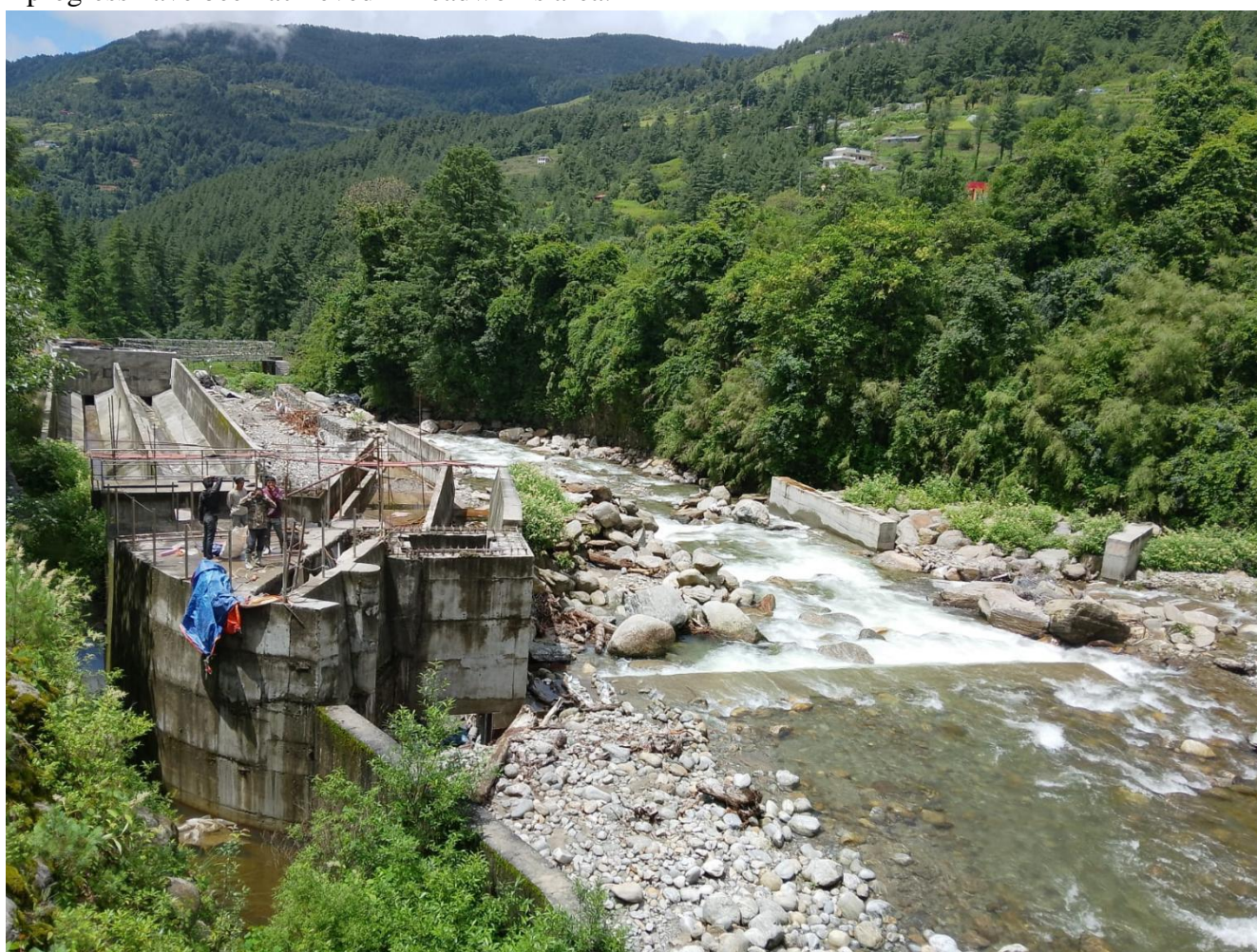
Figure 1:A view of headworks, showing weir, intake, gravel trap, settling basin, Viewing D/S.
