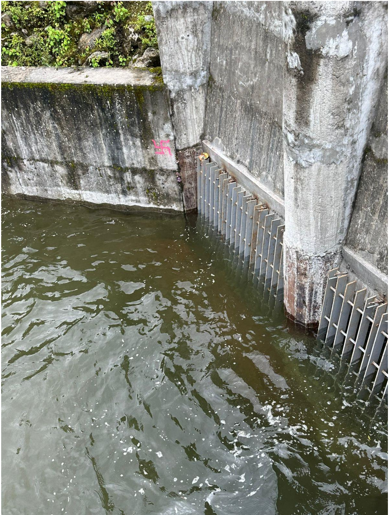
Figure 5:HM work progress ongoing Gravel flushing Gate frame installation work at site.
