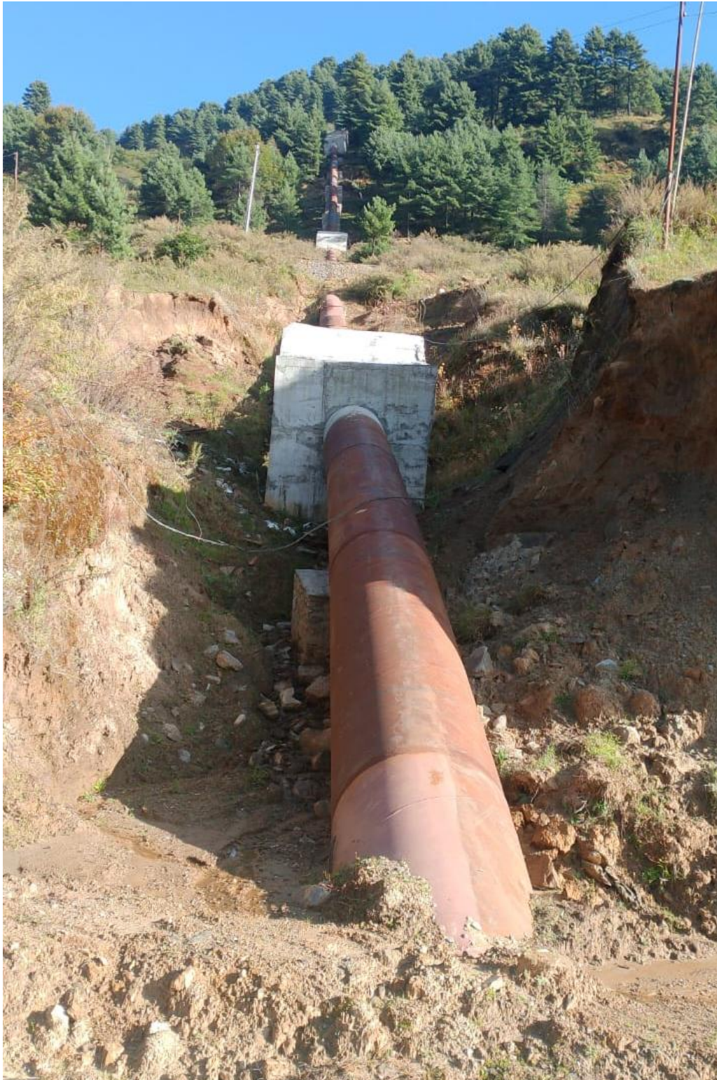
Figure 3: View of penstock after completion of erection, viewing U/S from Wyee Block.
